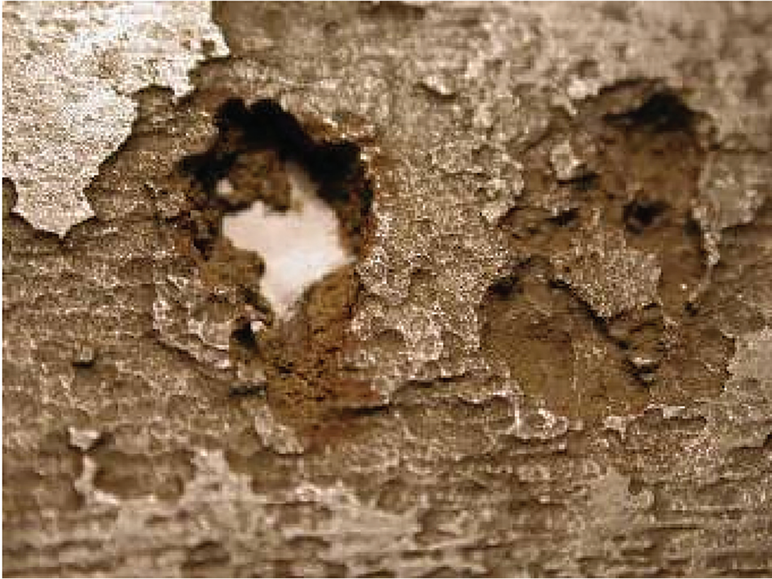
Fig. 5-6. Example of microbial corrosion (photo from Krieg, 2010).
