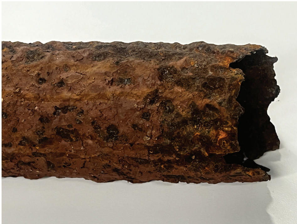
Fig. 5-2. Example of atmospheric corrosion (photo courtesy of Simpson Gumpertz & Heger).
