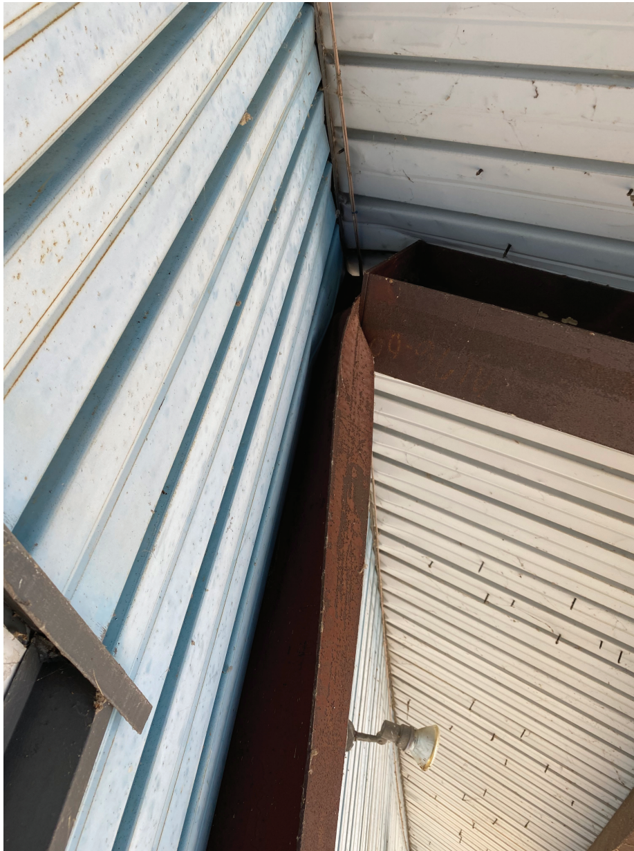
Fig. 3-4. Example of buckled roof framing (photo courtesy of Simpson Gumpertz & Heger).
