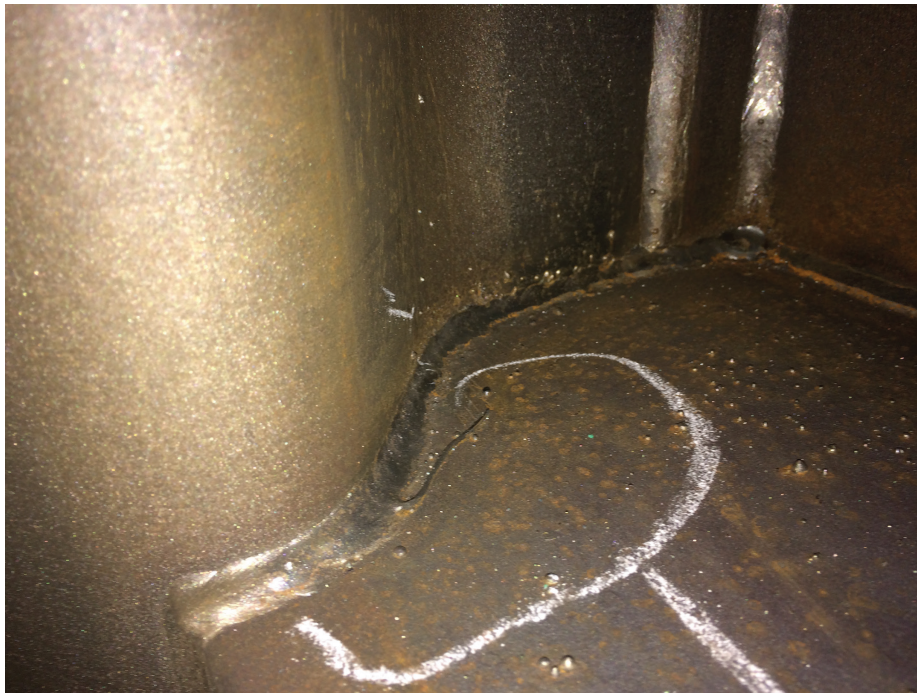
Fig. 3-3. Example of incomplete fusion (photo courtesy of Simpson Gumpertz & Heger).
