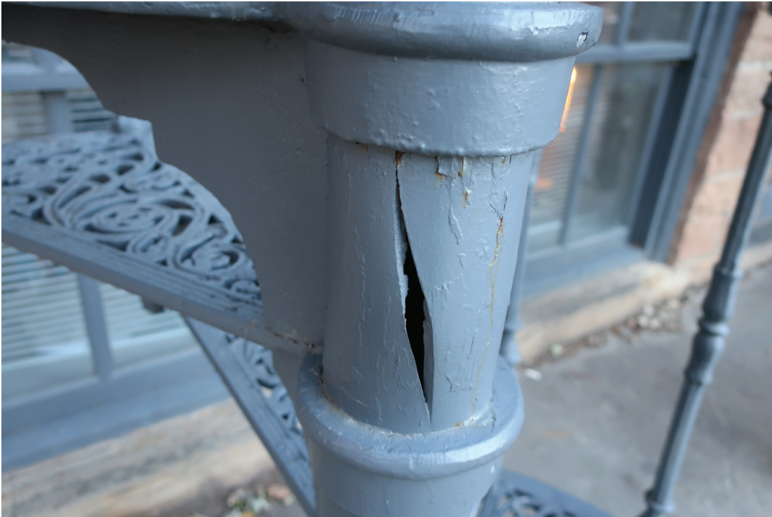
Fig. 7-1. Example of ice damage (photo courtesy of Simpson Gumpertz & Heger).
