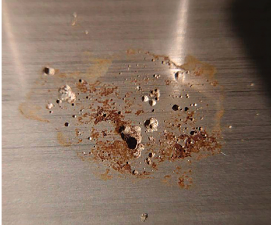
Fig. 5-4. Example of pitting corrosion (photo courtesy of Simpson Gumpertz & Heger).
